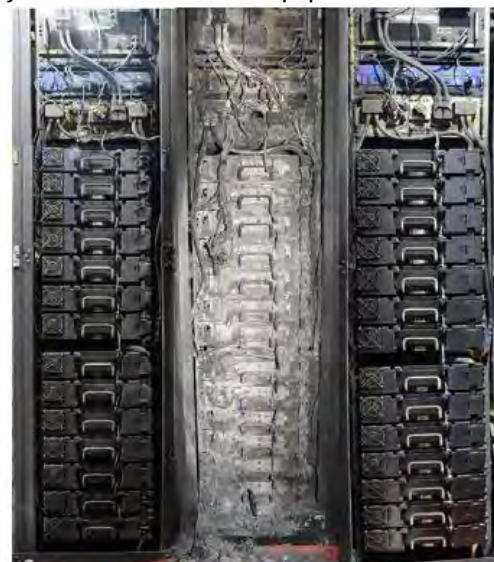
Rack 17 Rack 15 Rack 13
