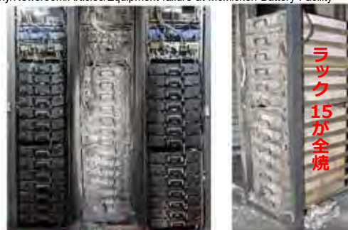
Rack 17 Rack 15 Rack 13
