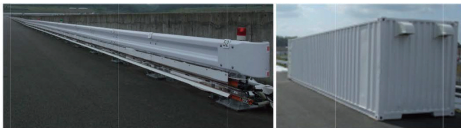
Figure 5. High-capacity storage battery and conductor rails
