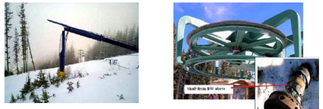
Fig.8 Tower break incident Fig.9 Bearing damage incident
